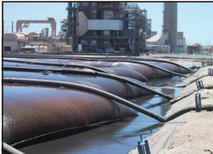
Geotube® containers at fossil fuel power plant being used to dewater fly ash.
