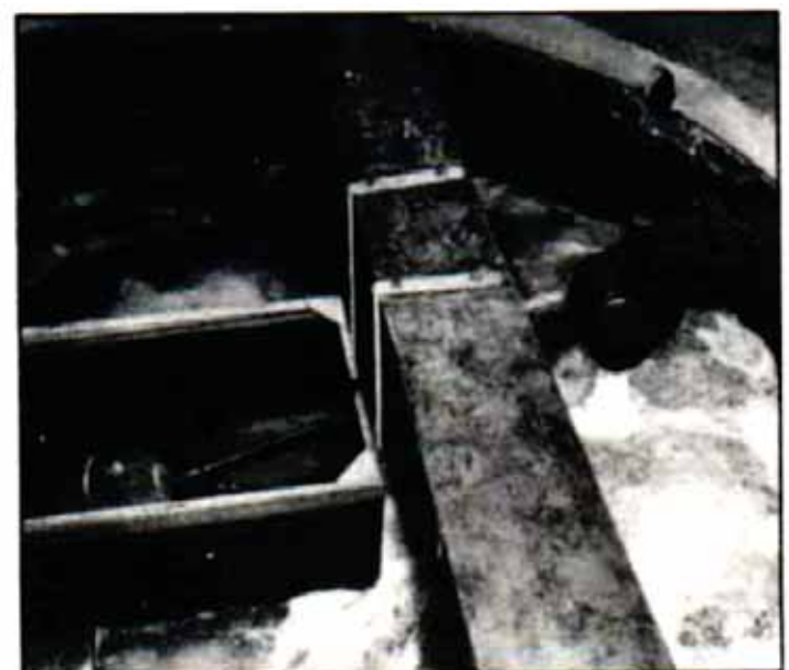
152mm inlet x 76mm outlet Larner-Johnson Float Valve on inlet to break pressure tank. This valve was installed in 1932 and has given continuous service without attention (barring dismantling for inspection and cleaning on one occasion during alterations to the system).
