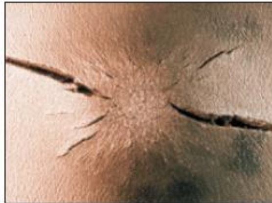
Fig. 11: Cracks at the inside wall of a PE 100 pipe subjected to an external point load and internal pressure (Test series 8)
